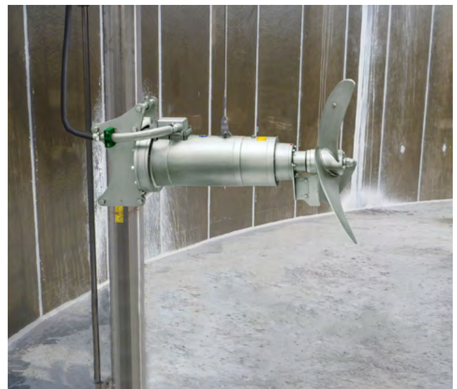
3A - Steel tank
