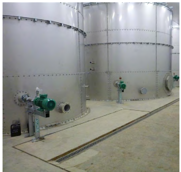
FR stationary - Steel tank
