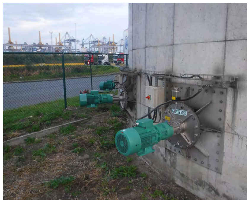
FR light - Concrete tank
