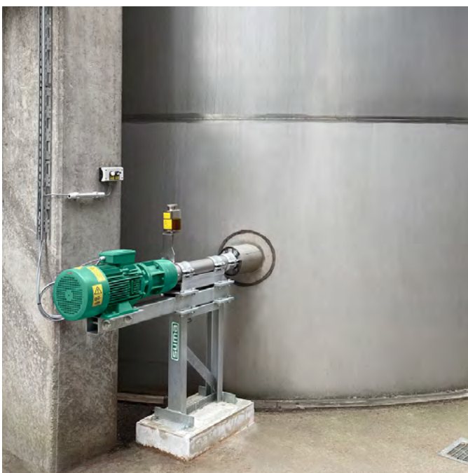
FR stationary - Steel tank
